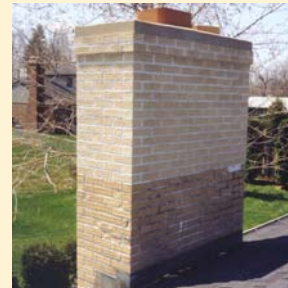
This partially rebuilt chimney would continue to deteriorate if left unprotected.
